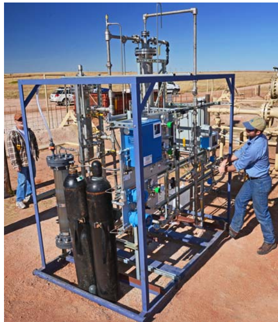
New Sky Energy's SulfurCycle natural gas scrubbing process is automated and monitored using Opto 22's SNAP PAC System control hardware and software.
