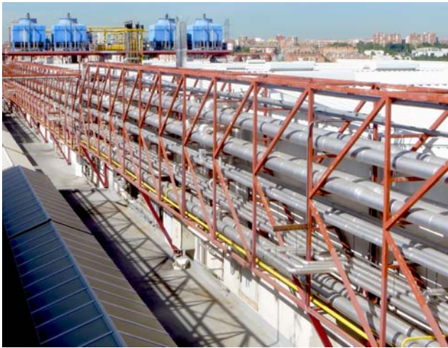
Liquefied ammonia, ethylene glycol, and other fluids are pumped throughout the market using a pipeline manifold equivalent to 43 mi. (70 km).
