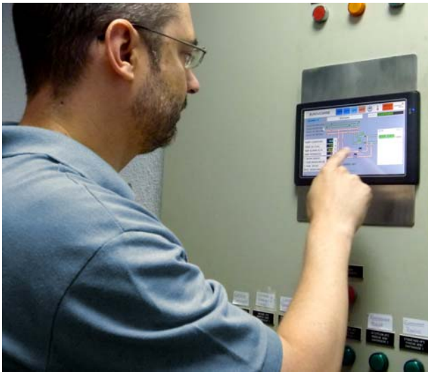
At each installation, each client can change setpoints, set alarms, and monitor temperatures for refrigerators and freezers using a local panel PC.
