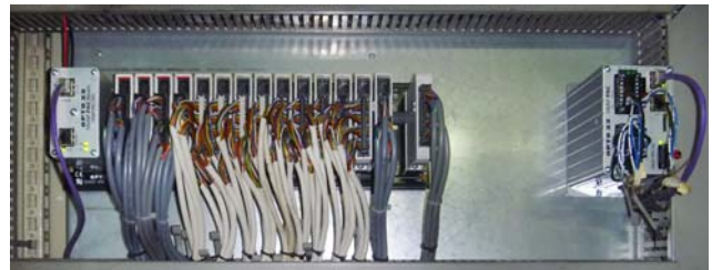
Original Telemechanique I/O hardware at the cold production plant was replaced with smaller Opto 22 SNAP I/O products. Special cabling reduced changeover time between control systems to minutes.
