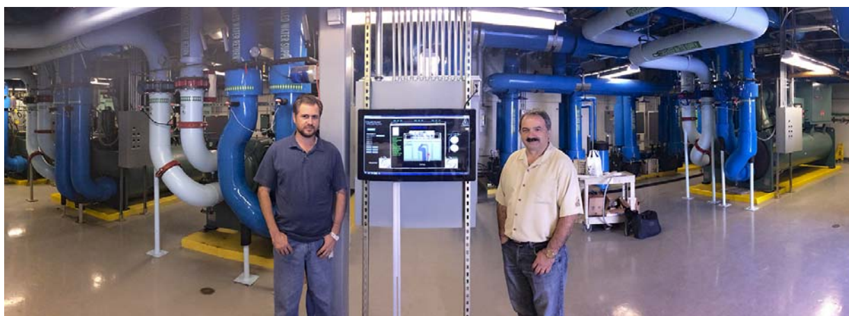
Carlos Terrazas (left) and Drazen Baricevic (right) with Arizona Facility Services (AFS) in the chiller plant of a retrofitted data center.
