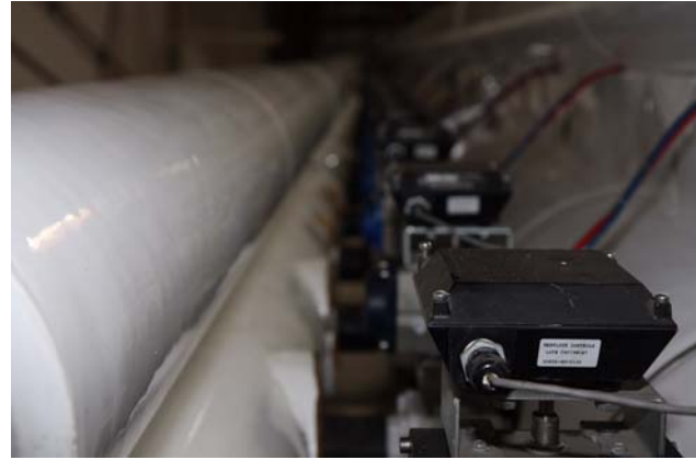
Multiple Opto 22-controlled valve actuators regulate delivery of hot water and liquid nitrogen needed for casting of the fiber optics
