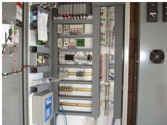
Racks of analog and digital I/O regulate many of the City of Carlsbad’s water-related activities.
