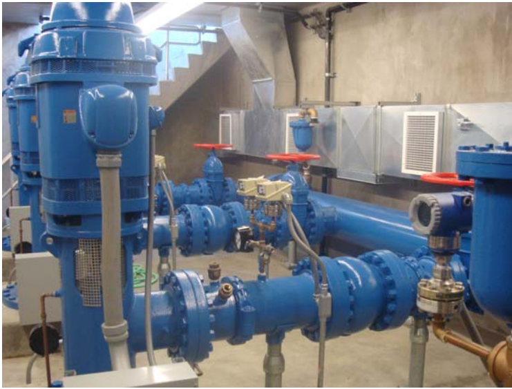
Pumps and valves at lift stations and booster stations are key parts of the city's infrastructure.
