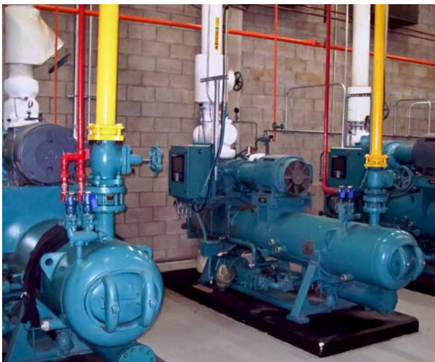
Systems integrator Advanced Energy Control designed and implemented a hardware system that intelligently controls SUPERVALU's refrigeration system, including compressors like the ones shown here.
