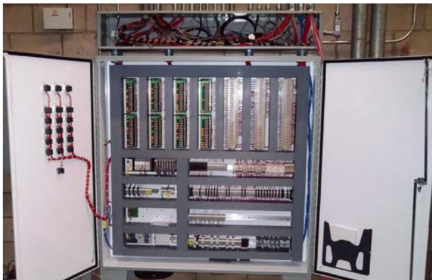
The OptoEMU Sensor and other SNAP PAC System hardware is wired to SUPERVALU's refrigeration system components and gathers consumption data that is then made available to both the company and curtailment service provider Net Peak
