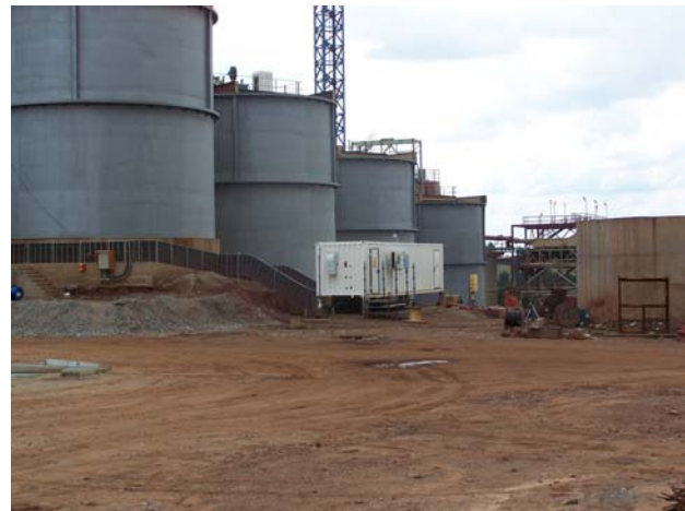
The Opto Controls control systems are located in large containers like this one in front of the large storage tanks.
