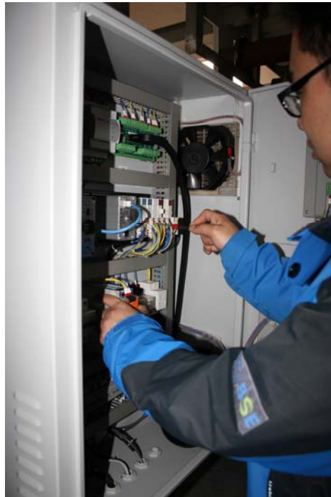
A BSE technician adjusts an Opto 22 SNAP PAC control system in a maglev chiller.
