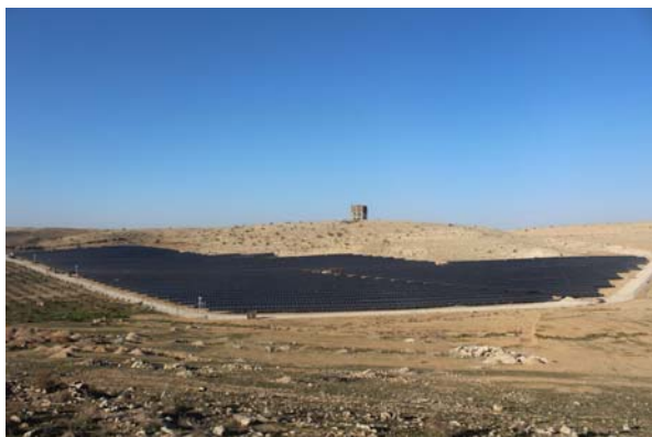
A 4 MW ground array provides the majority of the university's energy requirements.
